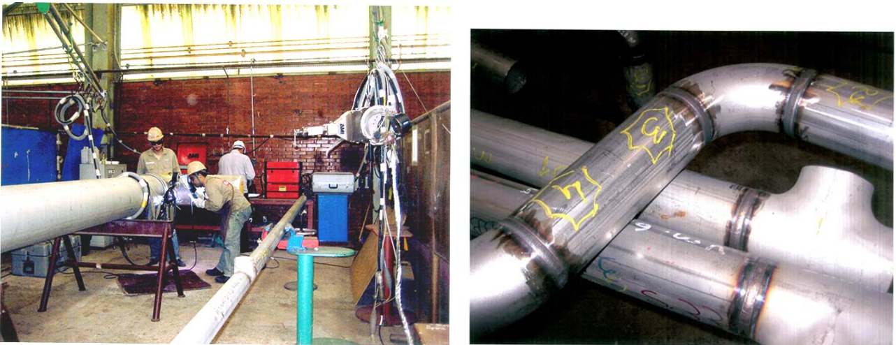
Figure 4. Left: Orbital welding of 2507 (UNS 32750) 20 inch duplex pipe with the AMI Model 15 and 4 inch pipe with the Model 79 weld heads in the prefabrication environment in the pipeshop at the BrasFELS Shipyard in Brazil. Right: Some orbital welds on pipe and fittings for the Petrobras P-52 Platform. Photos from Arc Machines, Inc.
